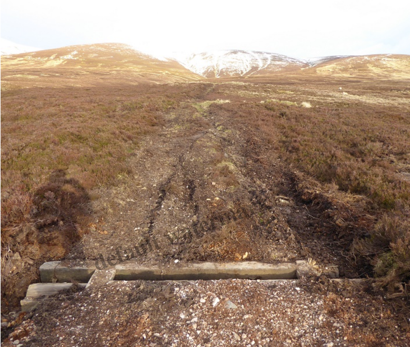
End of the 20m section of track showing erosion created beyond
