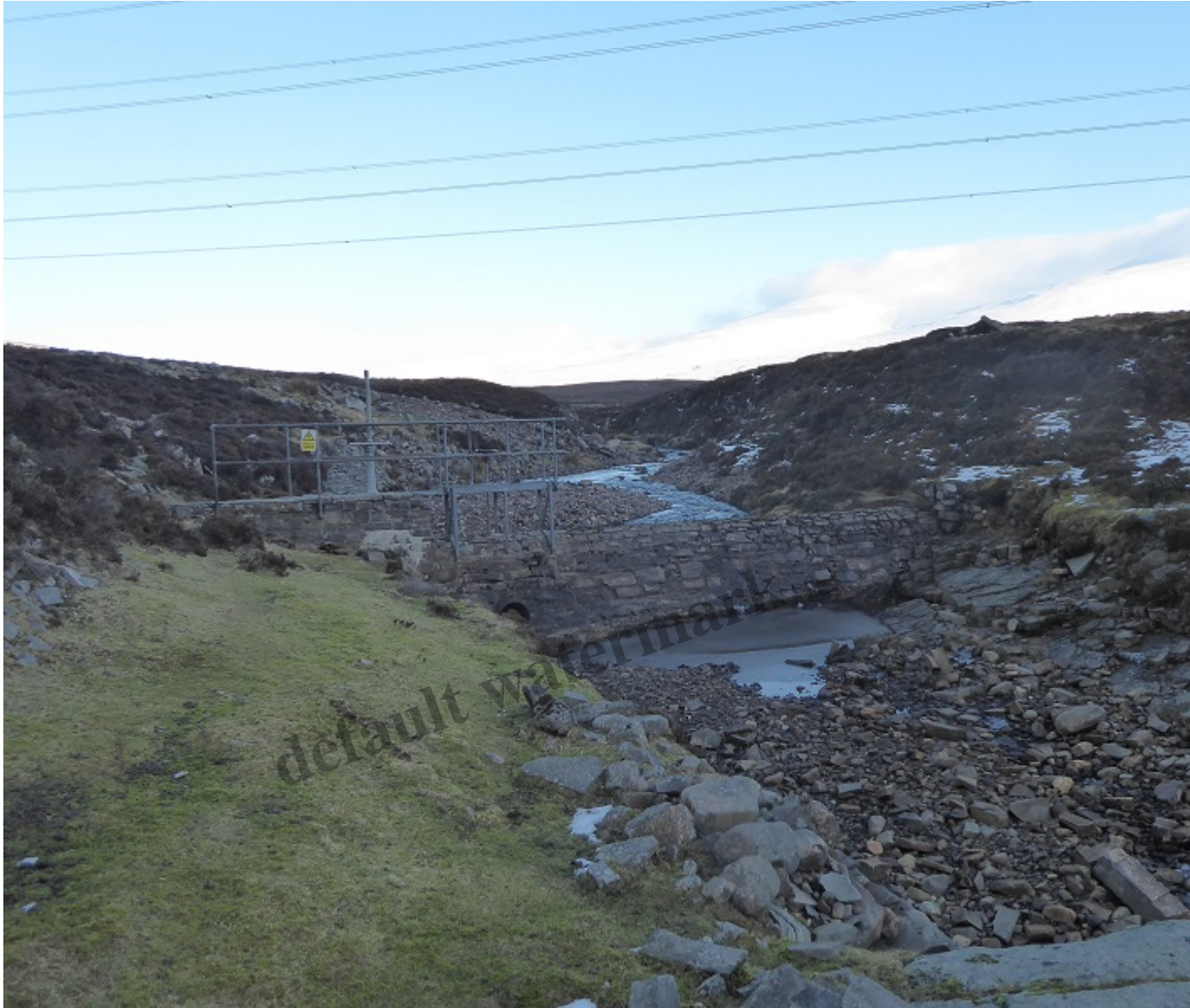
Stone faced intake, Cuaich hydro scheme, beneath Beaully Denny powerline, Drumochter.
