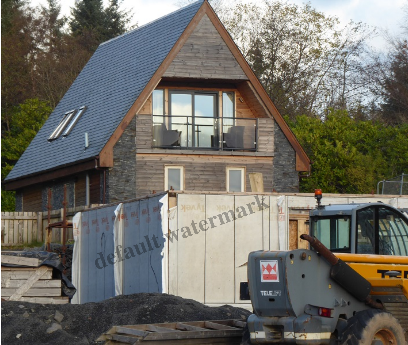
The very high specification storage shed – or as the LLTNPA described it Lodge No 15
