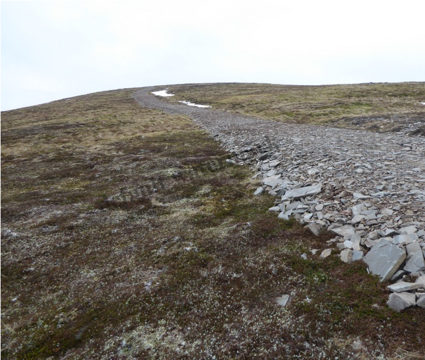
Top section of track onto Carn Leth Choin at head of Glen Banchor. The spoil has been dumped on windswept heath
