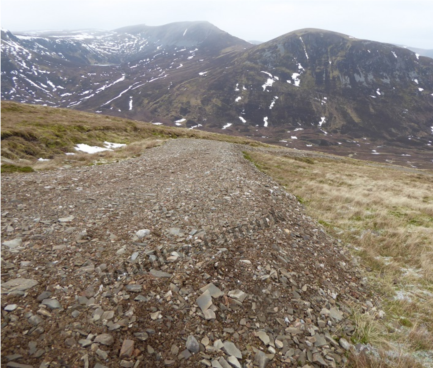
The section of track just above the large borrow pit. Loch Dubh in distance on left.
