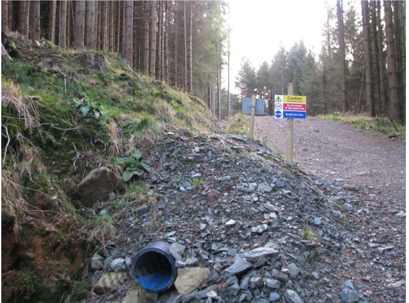
The poor finishing of culverts pictured here is evident in almost all the hydro scheme tracks in the Loch Lomond and Trossachs National Park. Photo Jane Meek.
