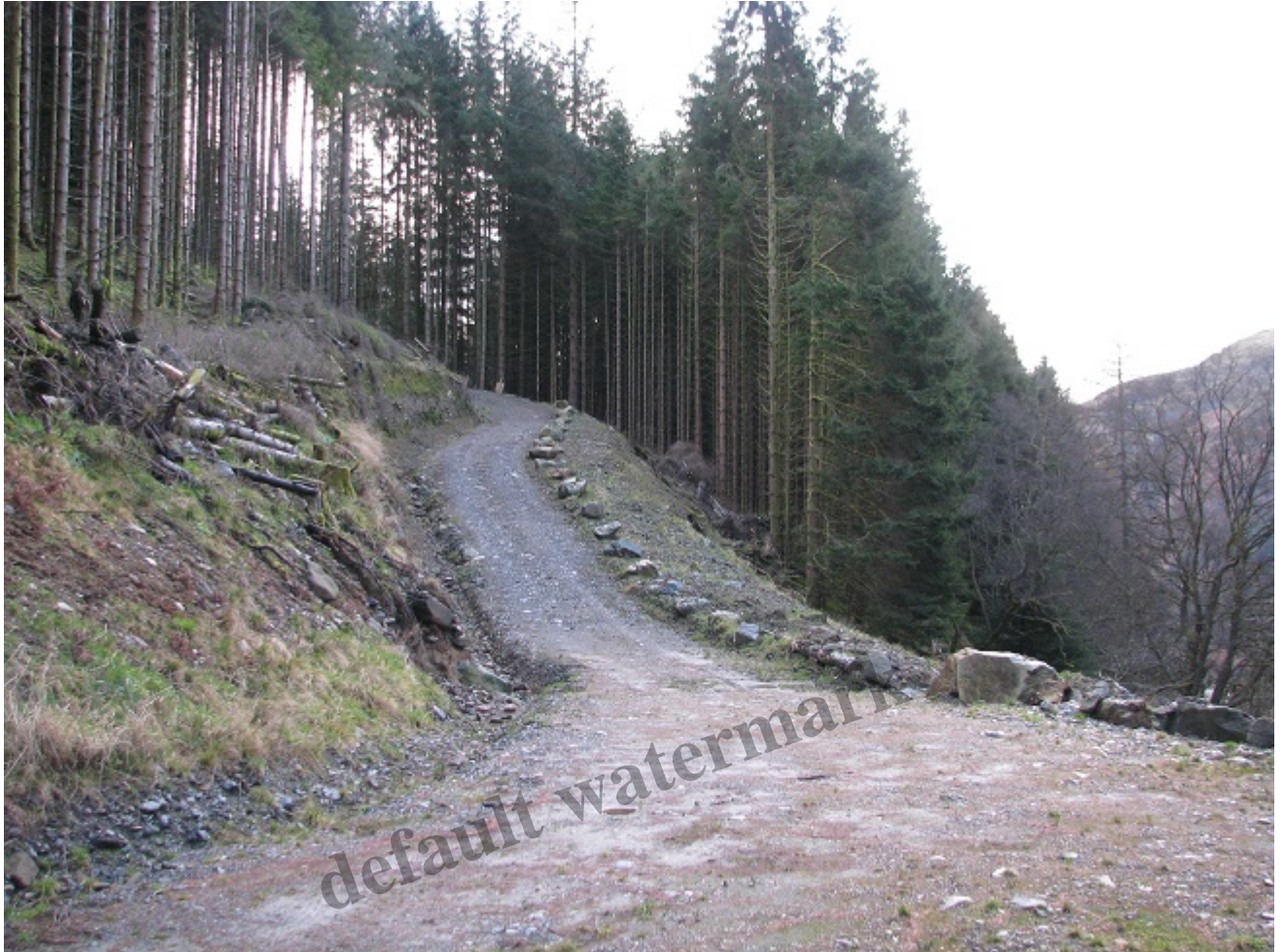
The new access track linked an existing track to the Ardchullarie intake (the hill path to Glen Ample is just beyond the end of the track in the photo). Photo Jane Meek.
