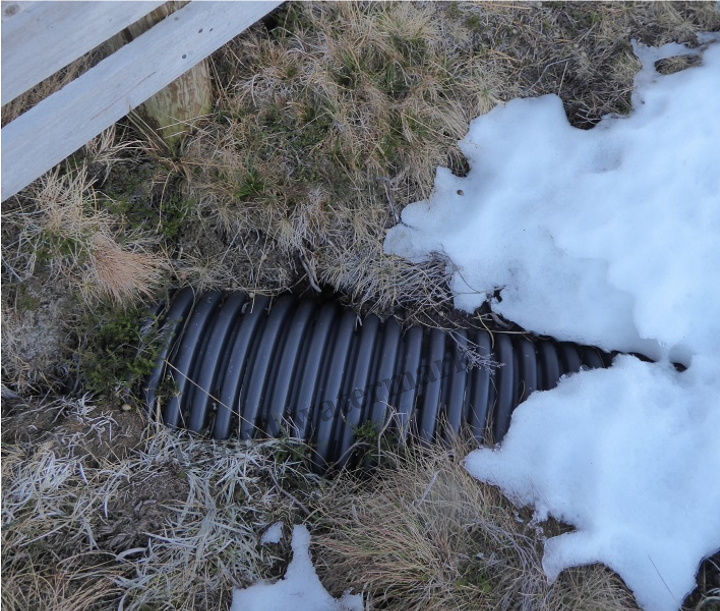
Section of poorly finished culvert crossing ski slope
