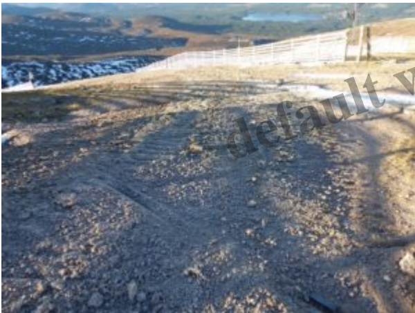
Choked drainage channel below Ptarmigan
