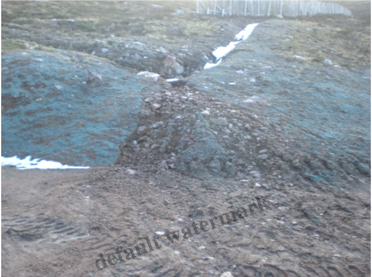
The ground to the right of the gantry, looking uphill showing where the blue revegetation pellets and topsoil have been washed away Photo Credit Alan Bratney 8/1/16
