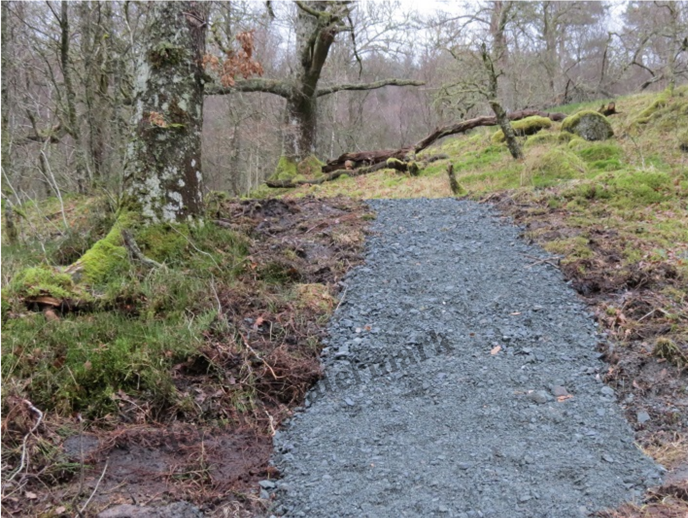
New track up to camping pitch. This track is almost certainly too steep and the aggregate is likely to
