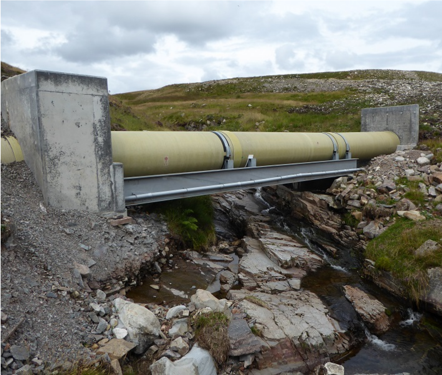
Pipeline – glass reinforced plastic – crossing burn just above power house
