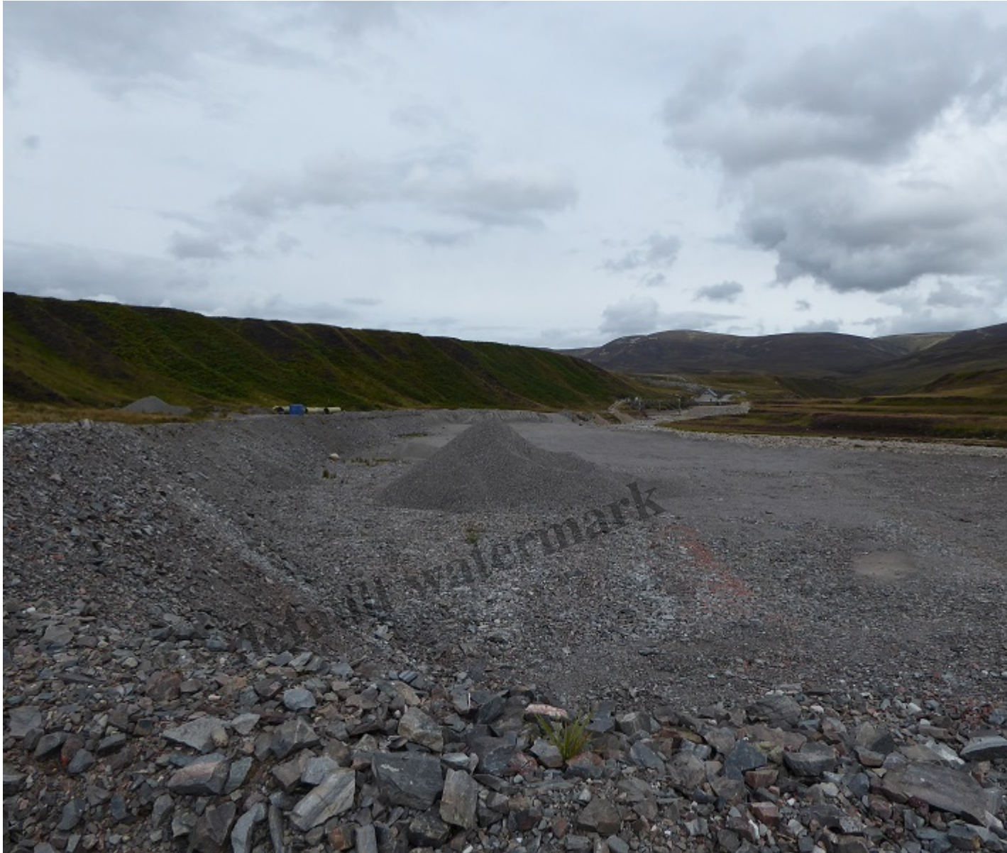
South of the powerhouse and the SSE intake is a large bulldozed area.
