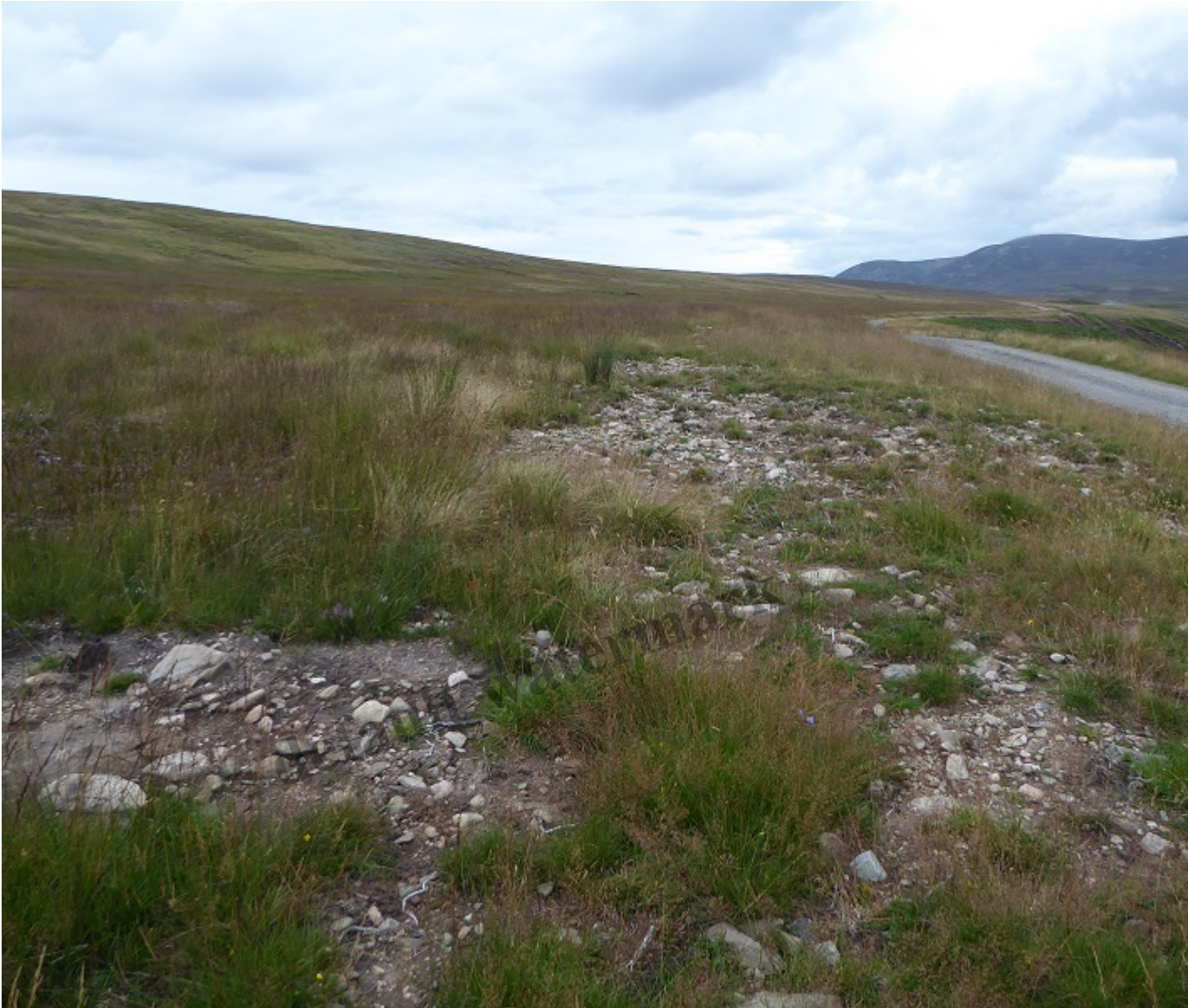
The new powerline runs alongside the existing access track from Calvine to Bruar Lodge.
