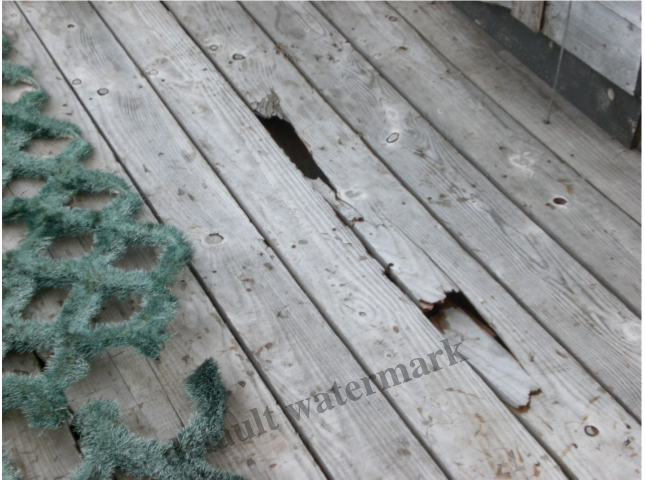
Loading ramp wood showing signs of rot
