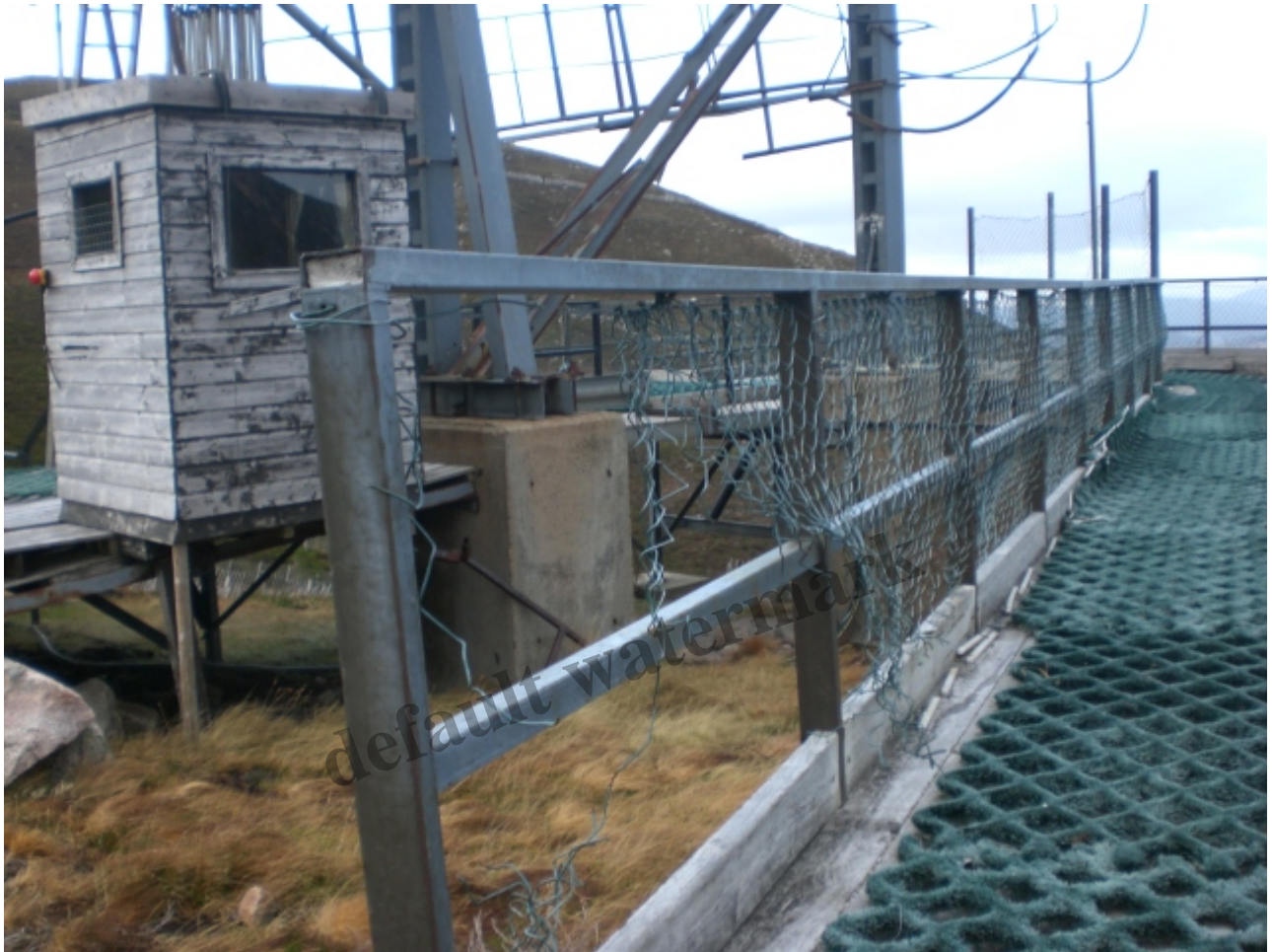
Loading ramp fencing in a dangerous condition
