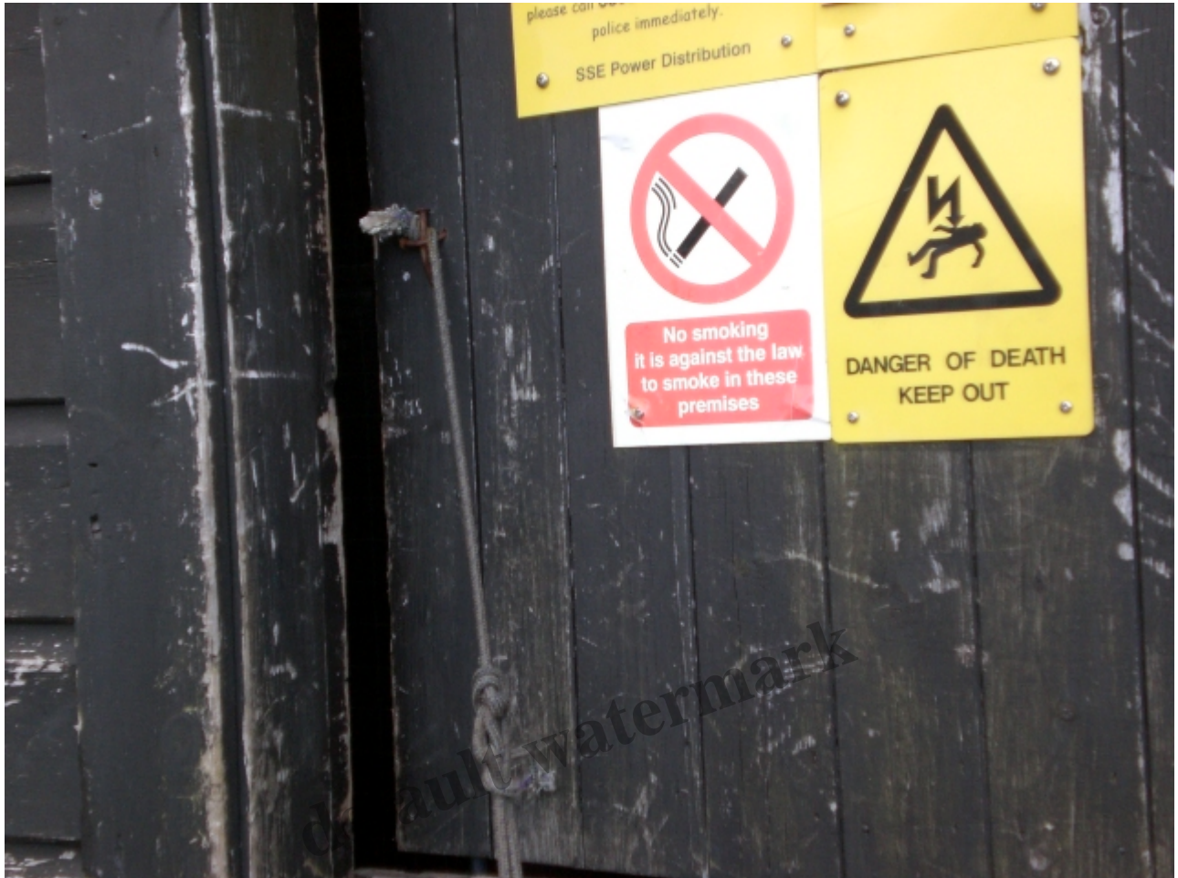
The control hut door does not close [tied together with twine but open enough to fill with snow in a storm. All photos Alan Bratney
