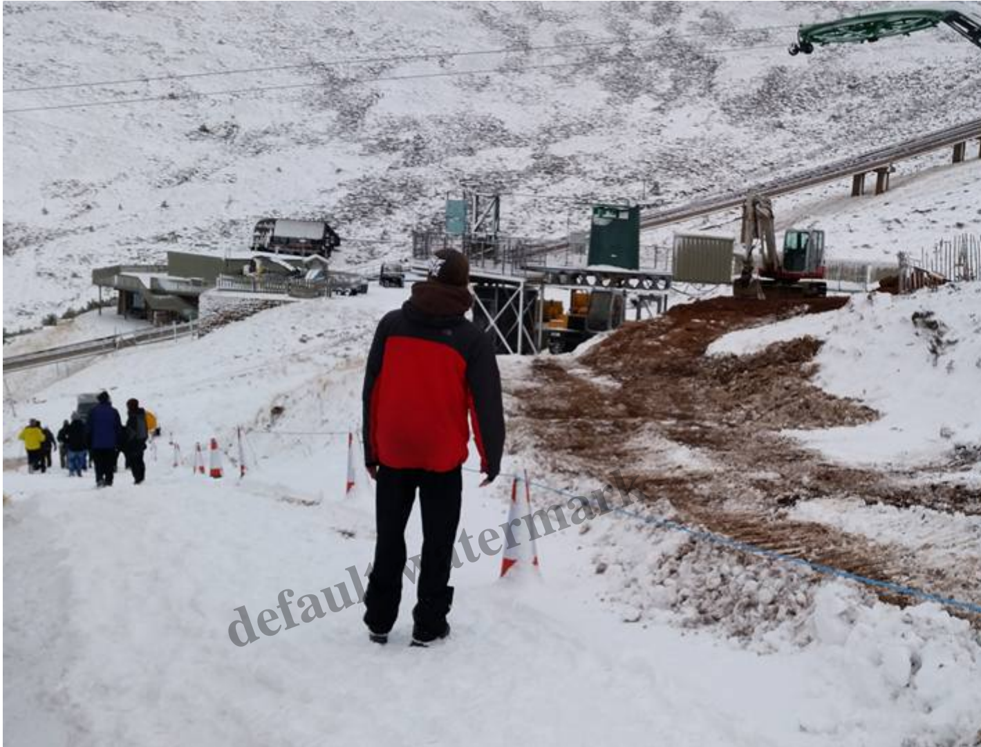
The initial works to “save” the Cas Gantry – Photo Credit George Paton
