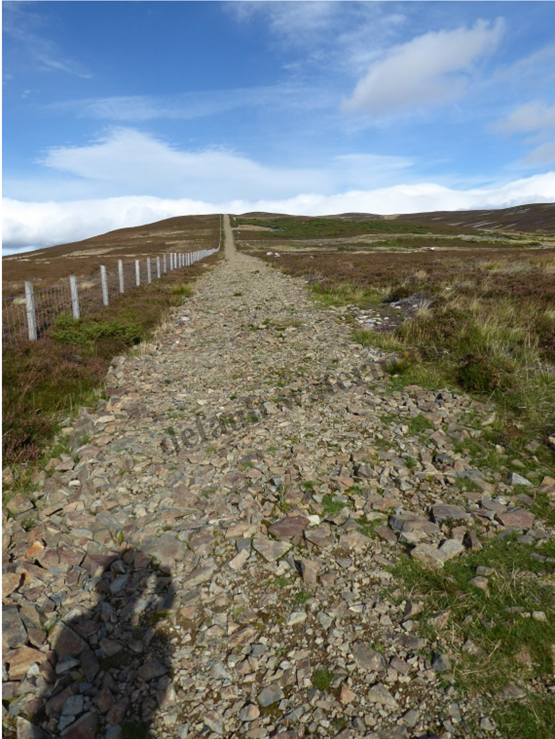
A closer view of track 1 from the start of the constructed section. The material for the track has simply been dumped on the moorland
