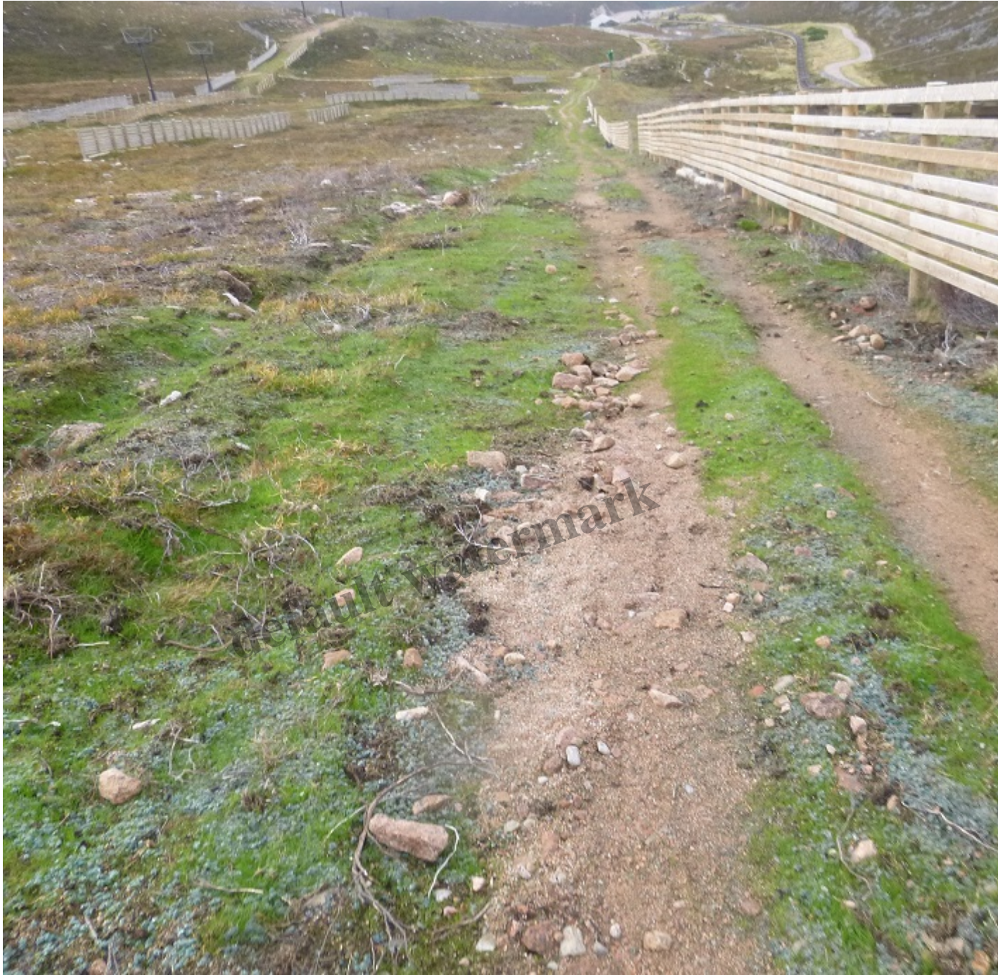
The steeper top half of the shieling track erodes each time there is a storm because its too steep and the track washes onto the surrounding re-seeded area Photo Credit Terry Smith
