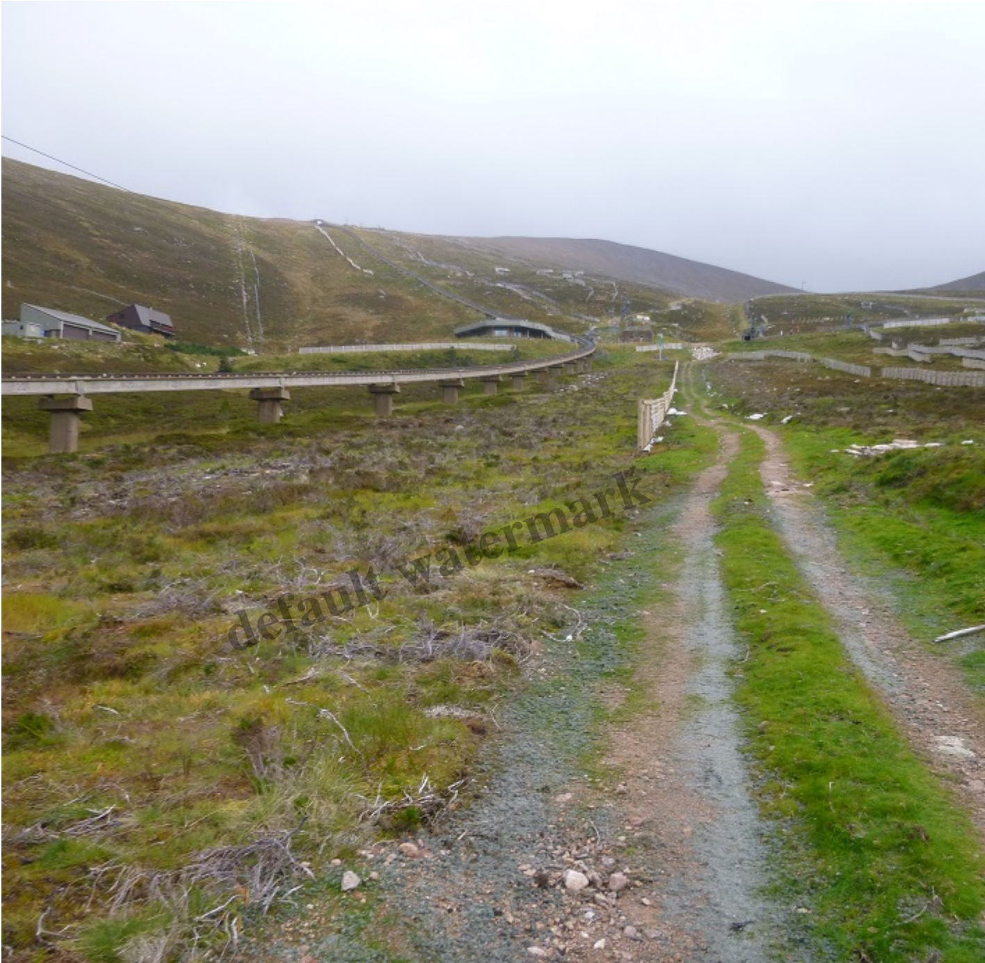
Half exposed pipes seem of no concern to the CNPA's landscape adviser
