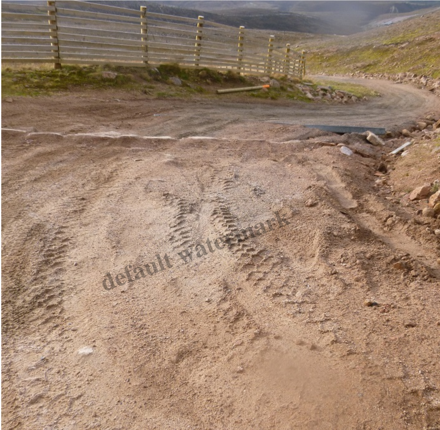
A lack of care in bringing vehicles up the mountain has damaged the access track. At one time per month a vehicle was taken up the hill.
