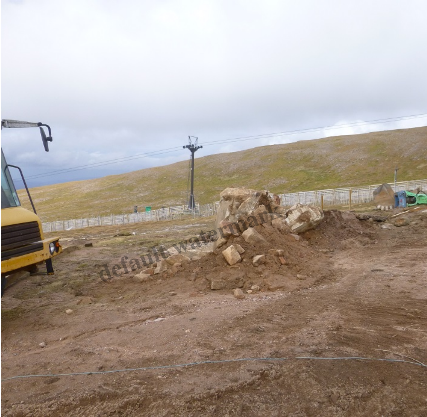
This aggregate is not being stored on matting as specified either. Dumping spoil like this simply dest vegetation.
