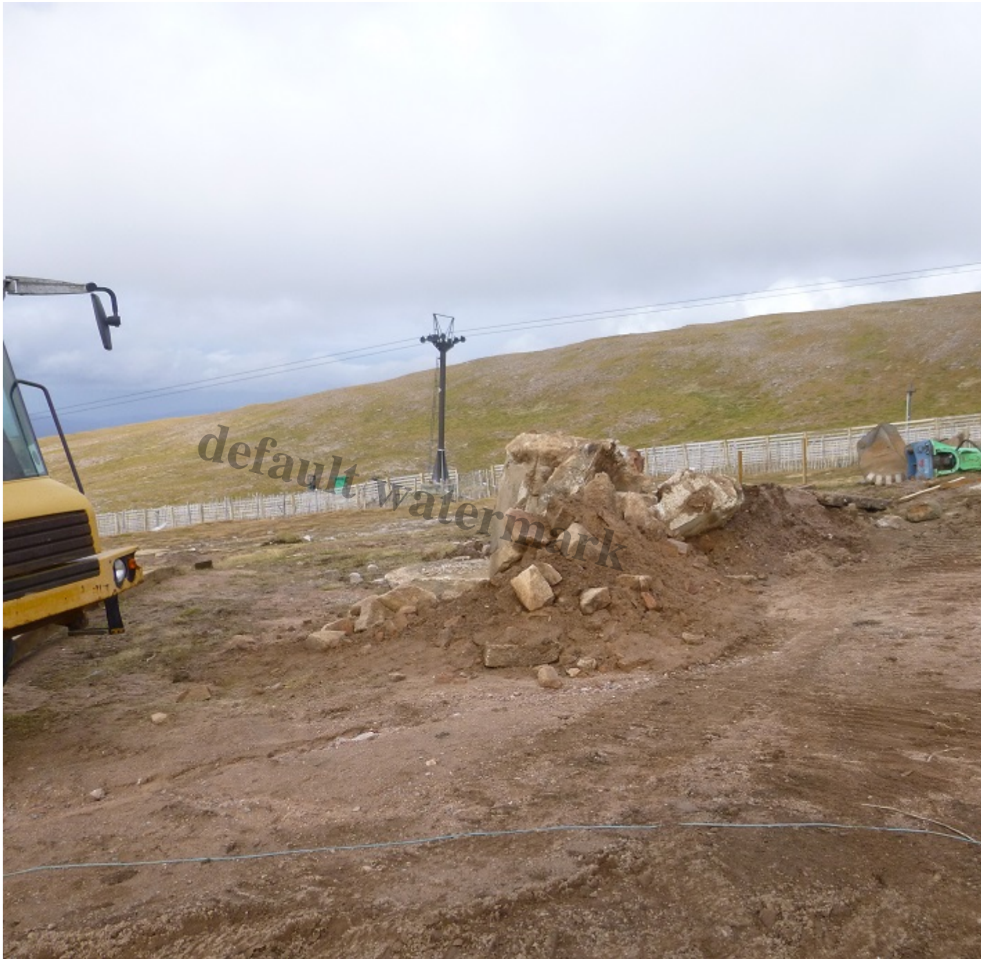
This aggregate is not being stored on matting as specified either. Dumping spoil like this simply destroys vegetation.
