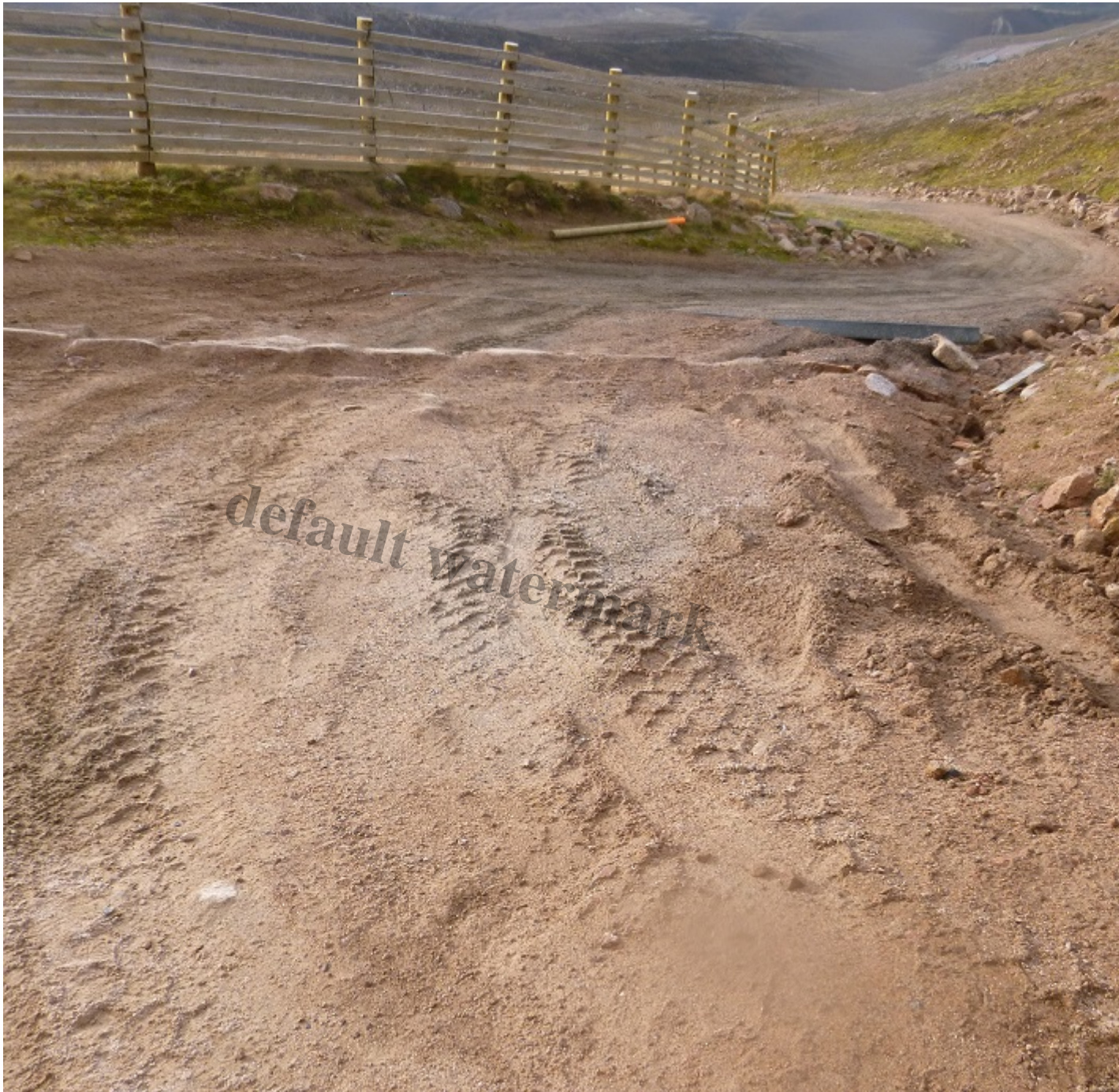
A lack of care in bringing vehicles up the mountain has damaged the access track. At one time per month a vehicle was taken up the hill.
