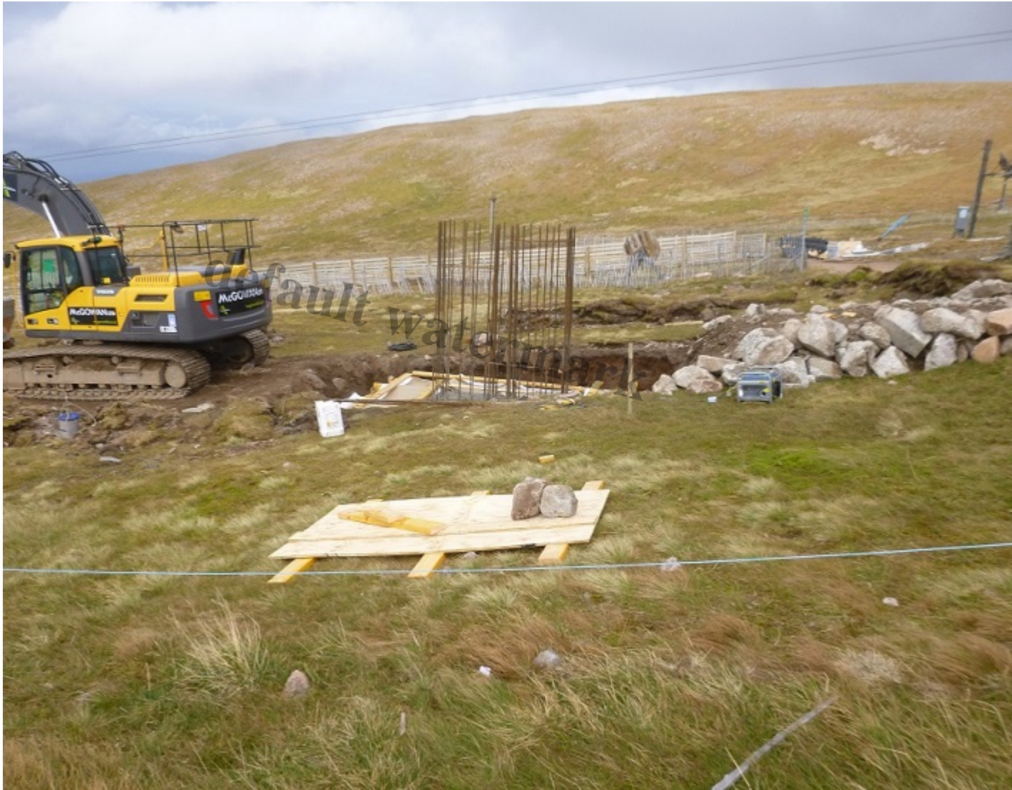
The foundations for the new fixed wheel at the top of the West Wall poma Photo credit Terry Smith
