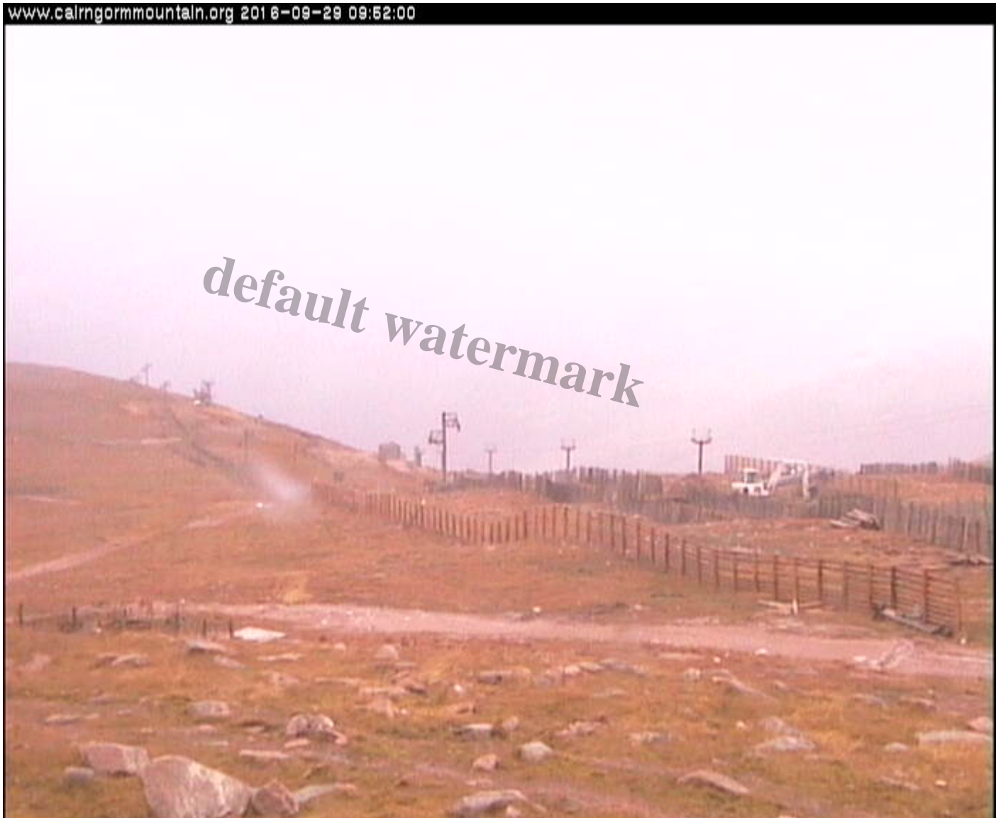
Digger operating outwith area granted planning permission â?? all vehicles were meant to be carefully controlled Photo from Cairngorm Mountain webcam (thanks to George Paton)
