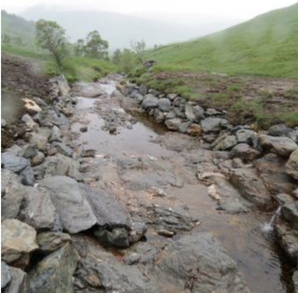
Rip Rap retention below Allt a Chuilinn intake – because the boulders have been built into the bank they have a lower landscape impact
