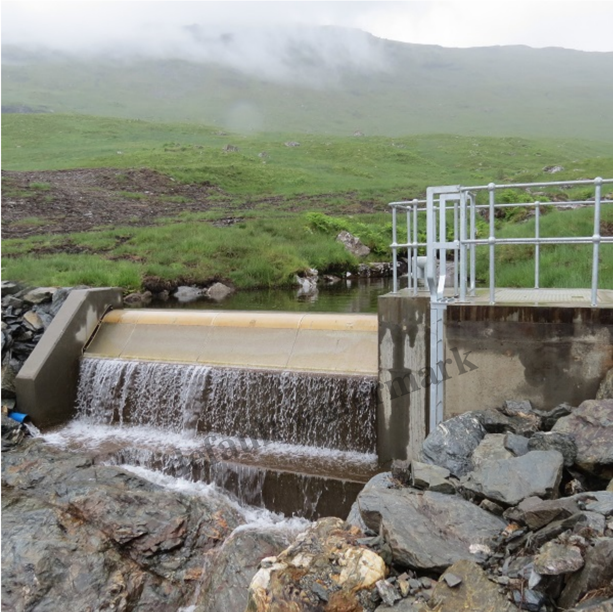
Allt Andoran – note boulders piled below right wall of dam and also lack of engineering of the pool behind – its looks natural
