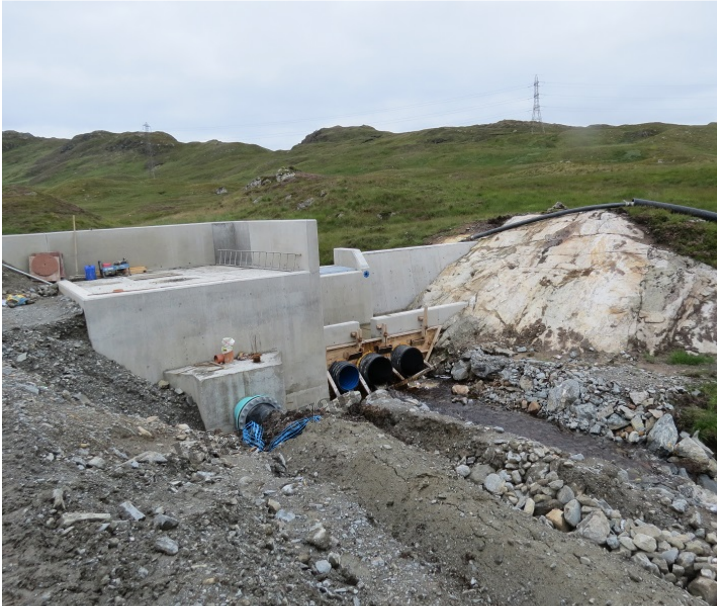
The first Ben Glas intake dam is located between natural features (moraine out of sight on left) but n has required significant amounts of material to be shifted and relandscaped.
