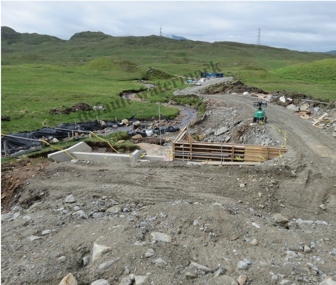
Photo illustrating how the second Ben Glas intake has been excavated out of the ground. The burn has been diverted temporarily to allow the dam to be constructed. The first intake is hidden behind the moraine of the track.
