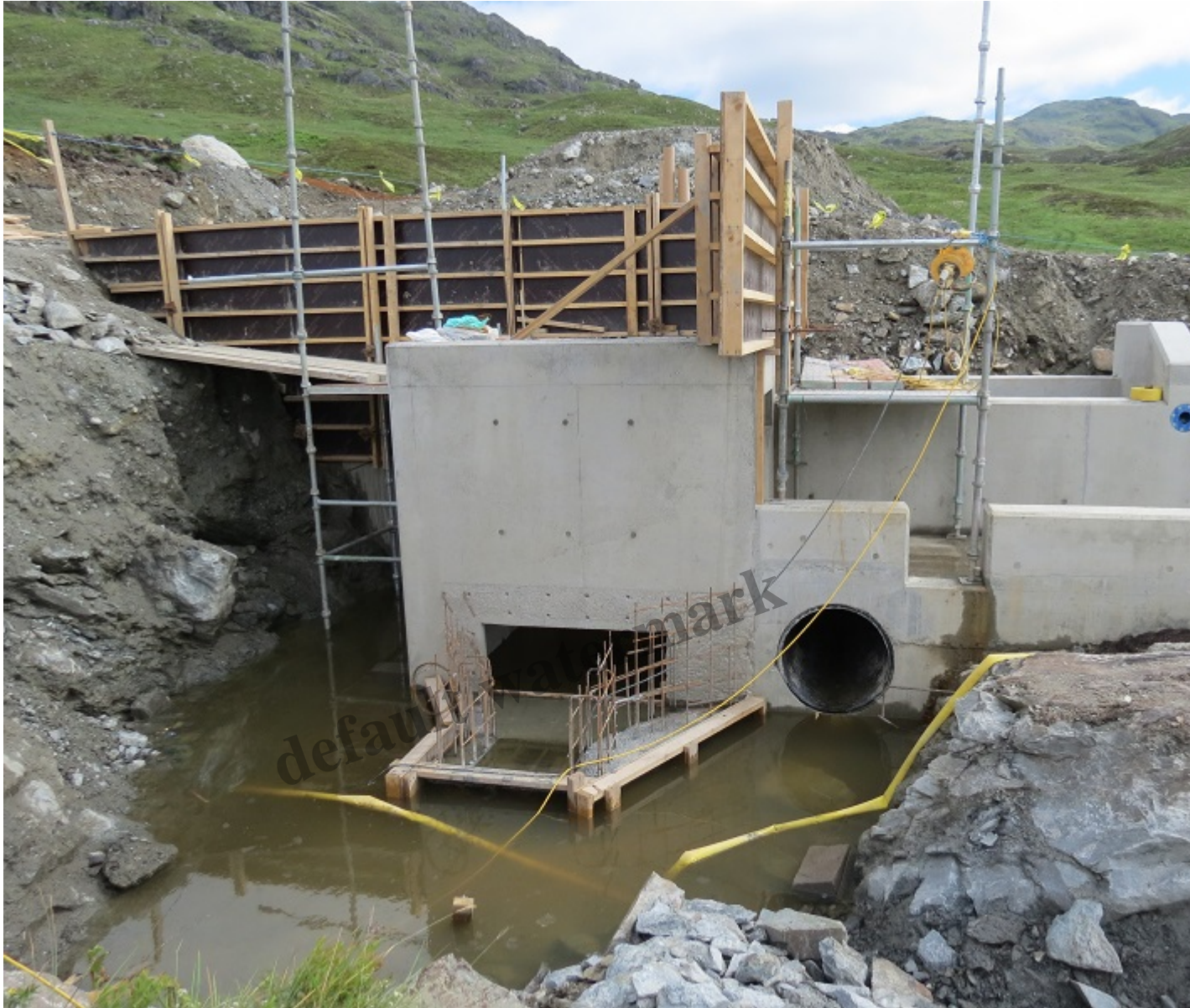
Second Ben Glas intake from below- significant amounts of concrete and other materials have been into what was once wild land
