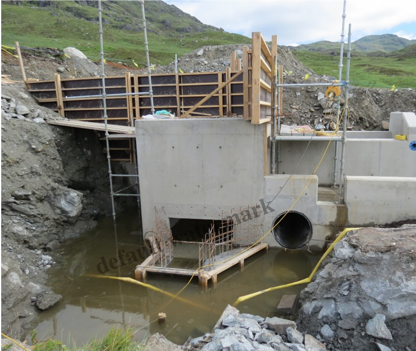
Second Ben Glas intake from below- significant amounts of concrete and other materials have been into what was once wild land
