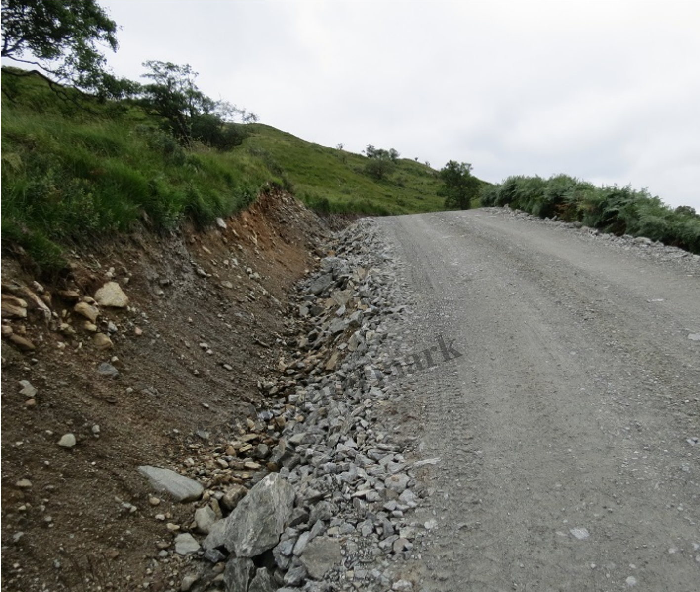
Part of the lower section of the access track to Ben Glas hydro scheme Glen Falloch illustrating the amount of aggregate used in its construction
