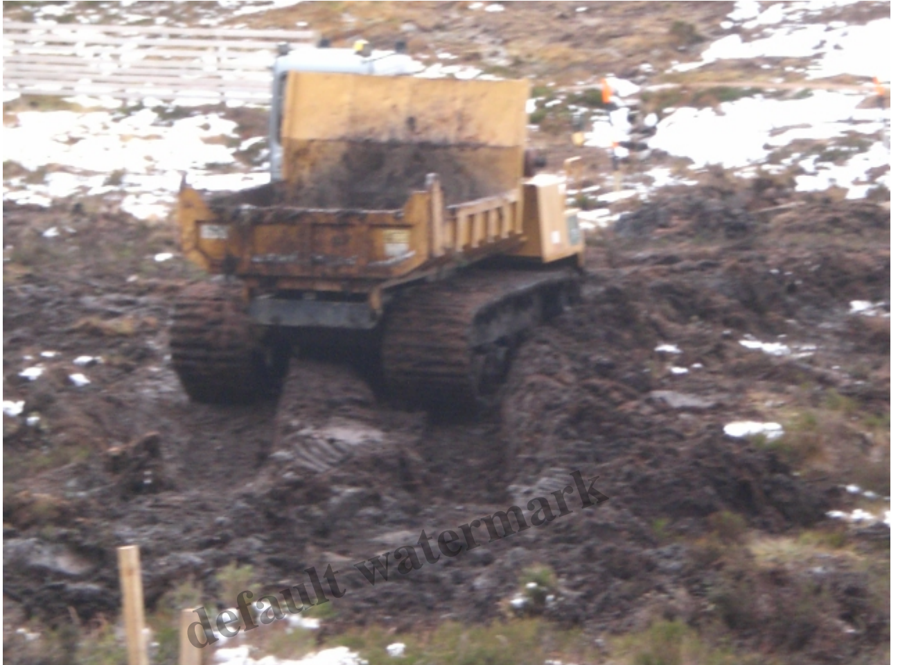
Construction vehicle bogged down in peat between the new track and the funicular Photo Credit George Paton
