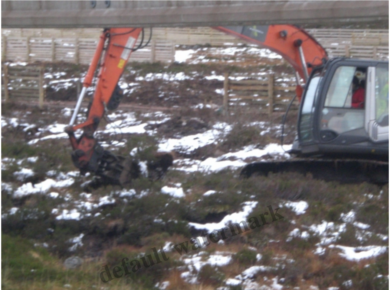
Digger ripping out vegetation (funicular support rail across top) having crossed ground that had been allegedly restored Photo credit George Paton
