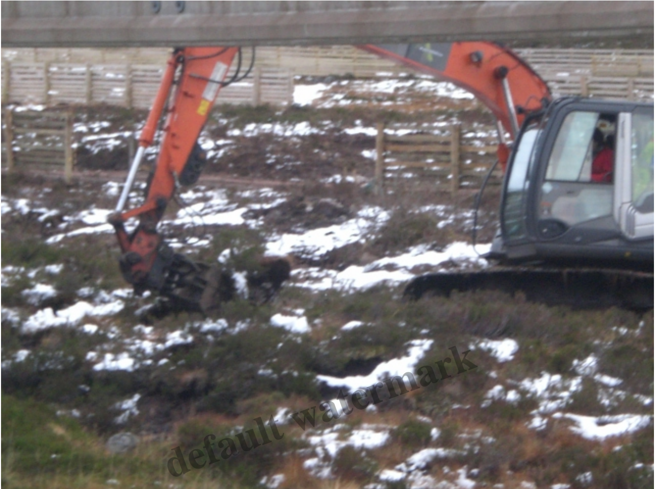
Digger ripping out vegetation (funicular support rail across top) having crossed ground that had been allegedly restored Photo credit George Paton
