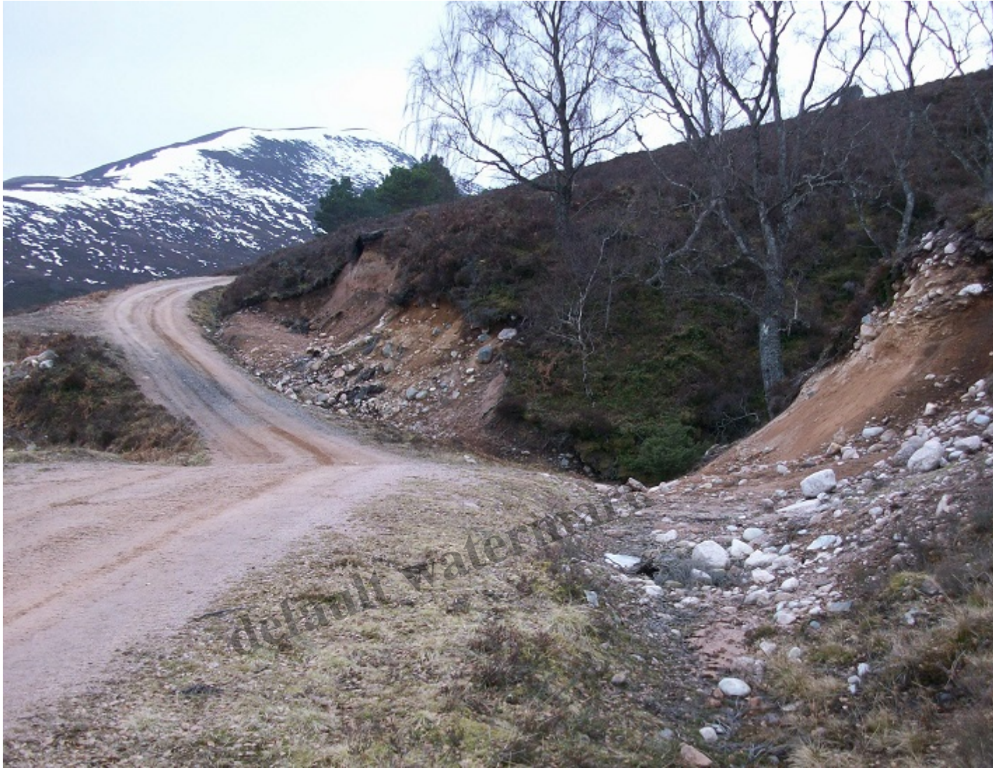
Poorly constructed hill track, Lynwilg, Cairngorms National Park Photo Credit Helen Todd
