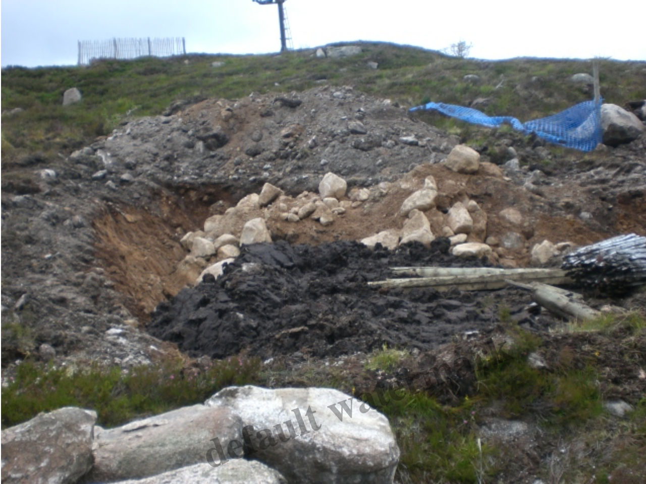
The backfilled hole – Car Park t-bar in background Photo Credit Alan Bratney
