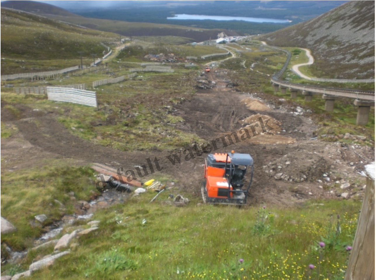
Work in progress on the Sheiling Poma 29th August 2015. Photo credit Alan Bratney
