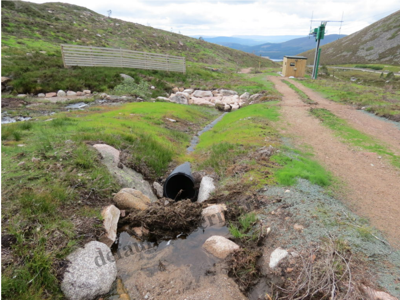
One of two unfinished culvert on the edge of the Sheiling Poma ski slope – there are three culverts in all, only two of which are referred to in the planning application
