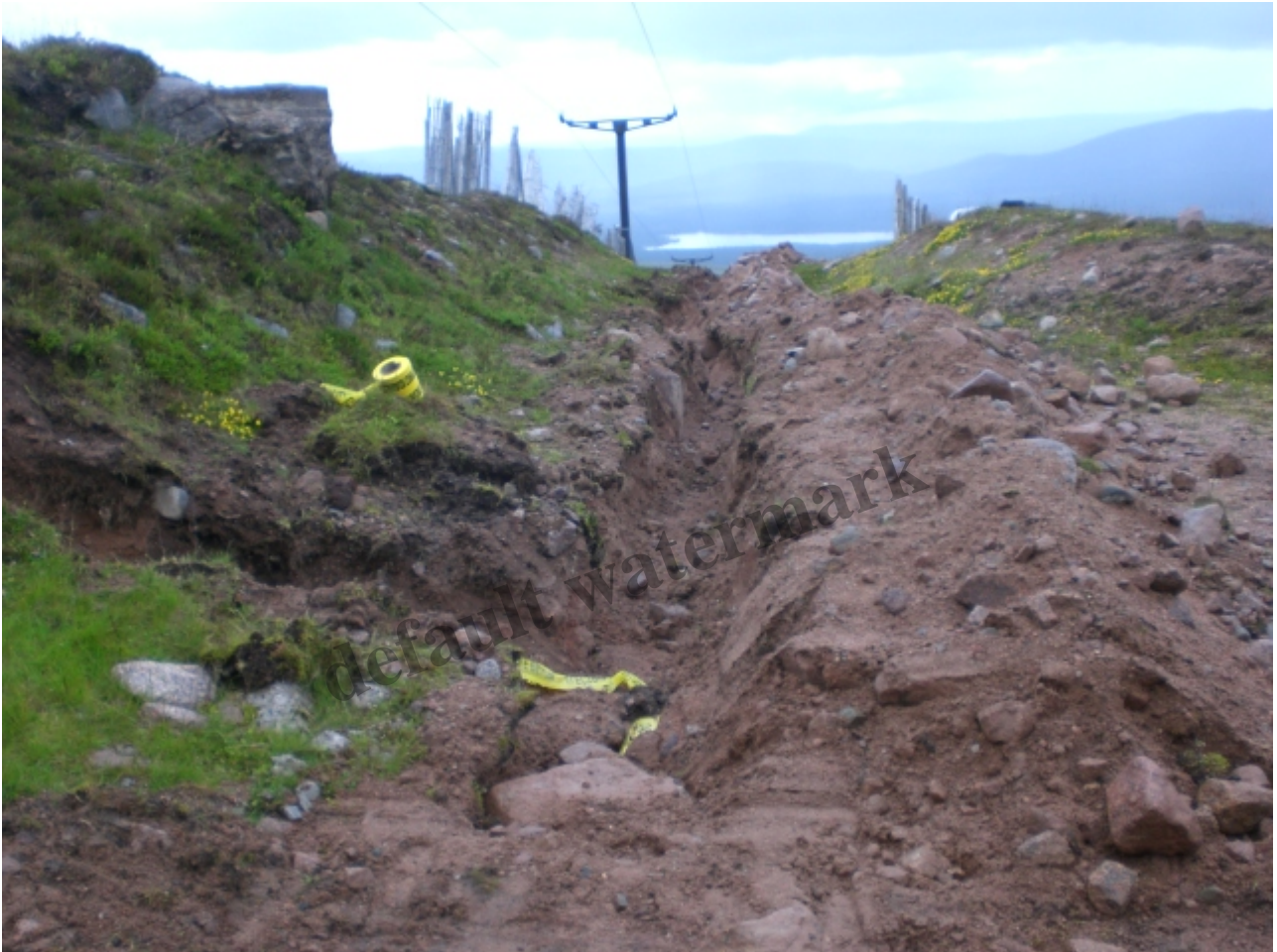
The trench that has been dug along the entire length of the car park T bar to install new cabling – photo credit George Paton
