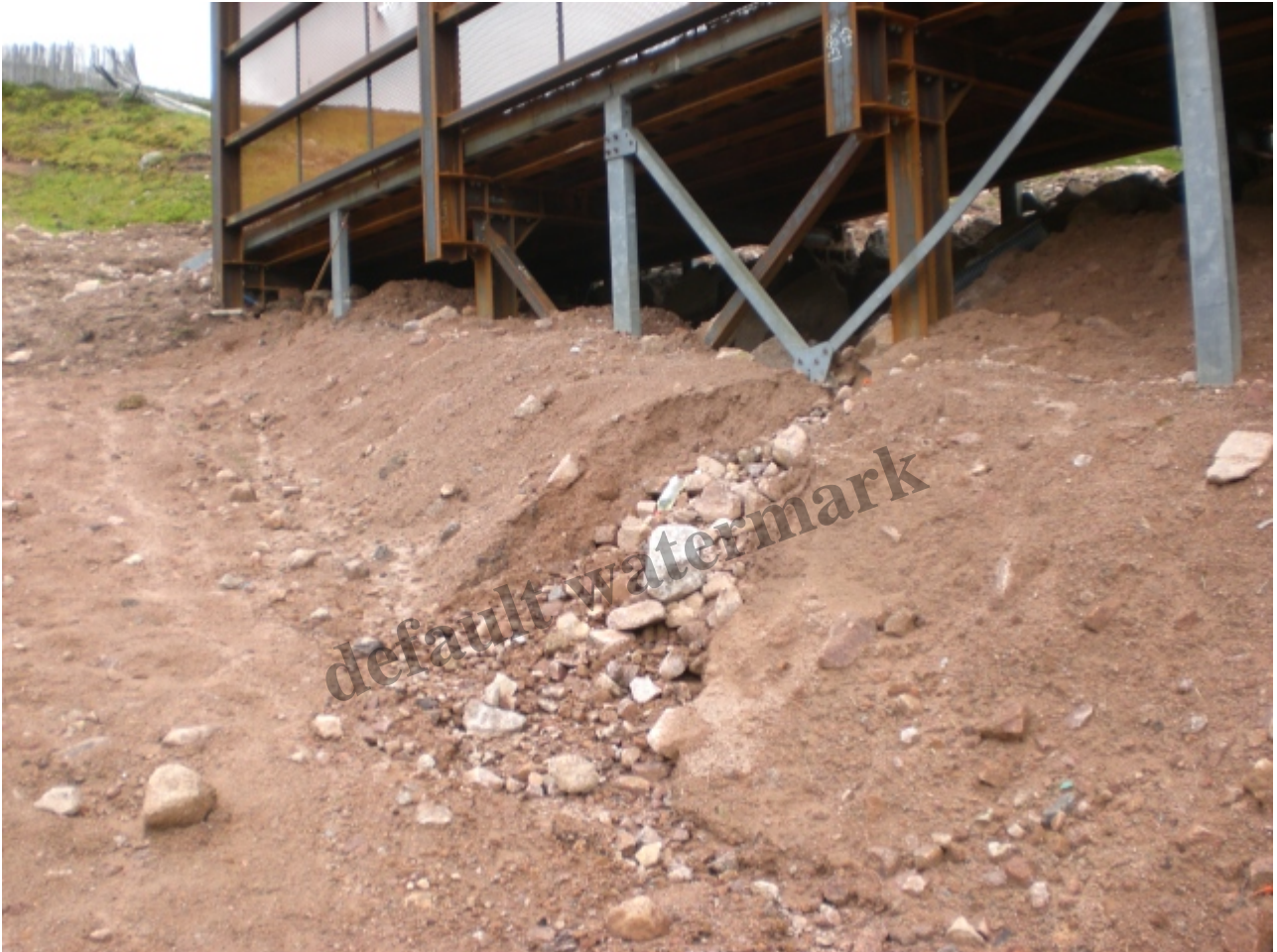
The new Coire Cas T-bar platform with spoil below. It is already being eroded away by the rain. Photo Credit Alan Bratney
