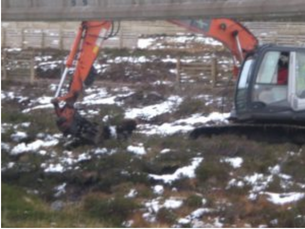
Digger operating outwith area granted planning permission – the lack of boundary markings made it easy for them to do this
