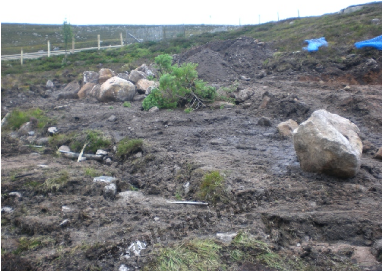
The Method Statement did not say what would happen to boulders that impacted on the “reprofiling” of the slope Photo credit Alan Bratney
