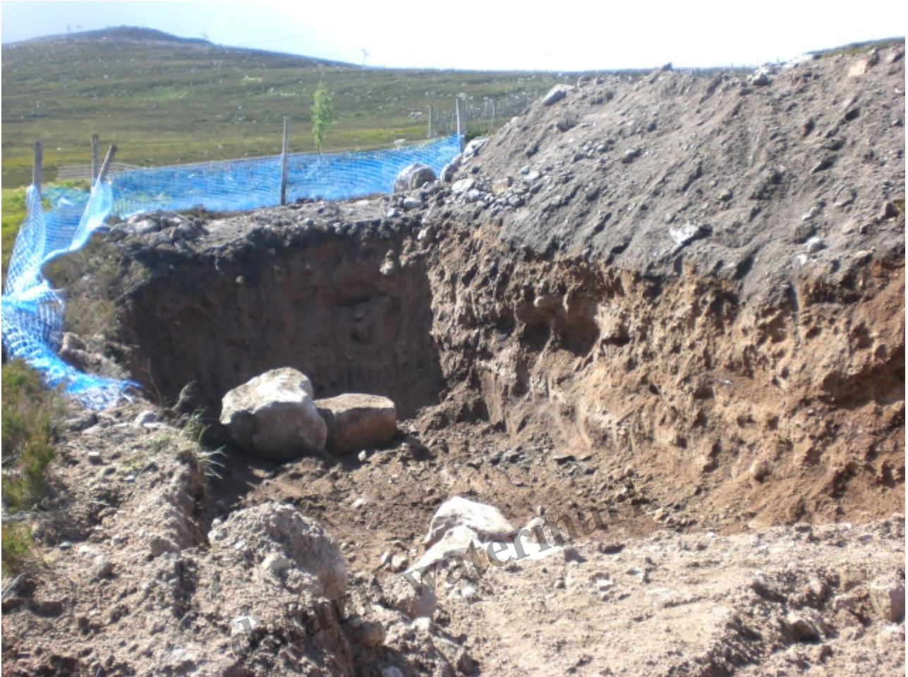
Pit into which soil, peat and boulders was later dumped Photo Credit Alan Bratney
