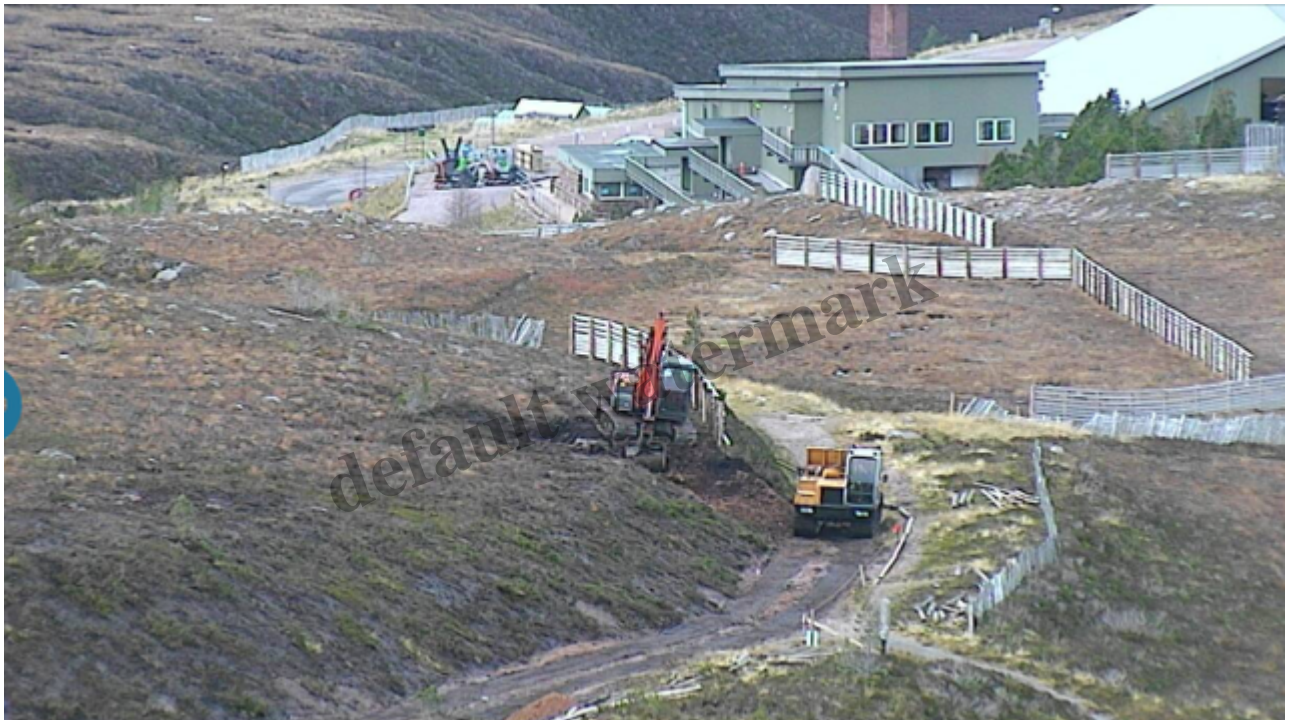
Working taking place on the bank below the shieling ski tow – the planning permission did not cover this area credit George Paton
