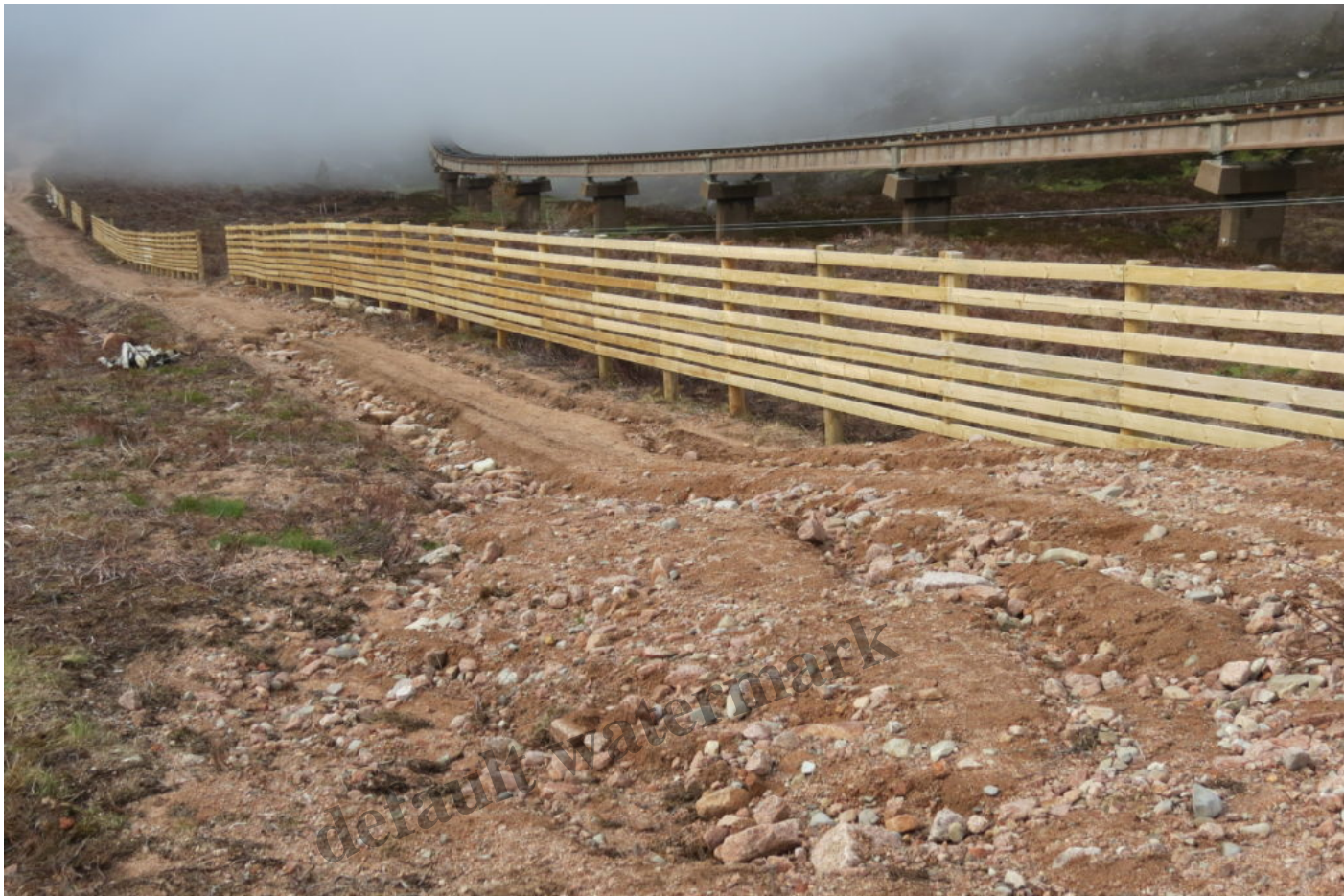
Erosion, including gullying at the top of the new bulldozed track
