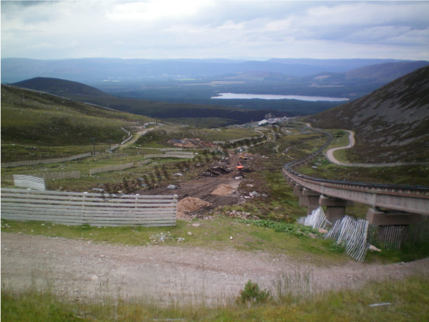
Photo credit Ron Greer. Bulldozing ground lower Coire Cas before installation new ski tow and snow fencing
