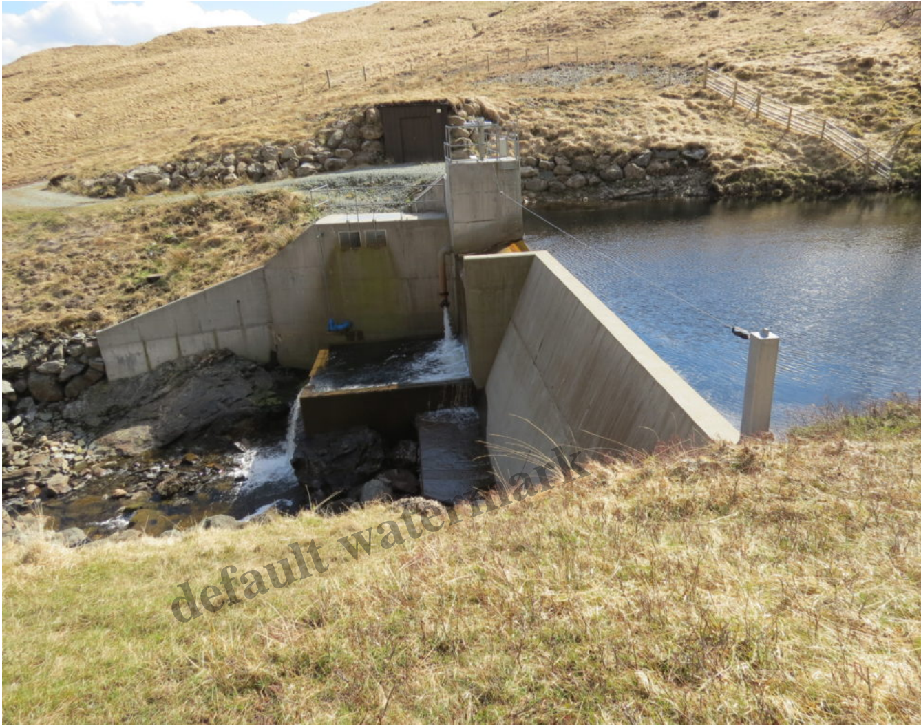
The Allt Fionn dam on northside of Glen Falloch. The dam is well situated at bottom small gorge and almost invisible from above until close to it and the main visual impact is the dam itself.
